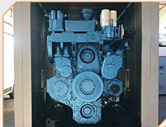
DANIELI AUTOMATION 2250KVA - CONTAINER PRP - CINA
